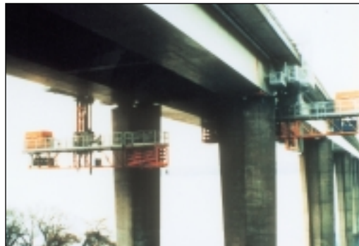
Inspection and Maintenance Platform, Tay Road Bridge. OEM: Monkcradle.
